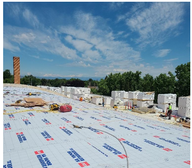
July 7 – Roof work ongoing at Baker Middle School Gym as part of seismic upgrades.
